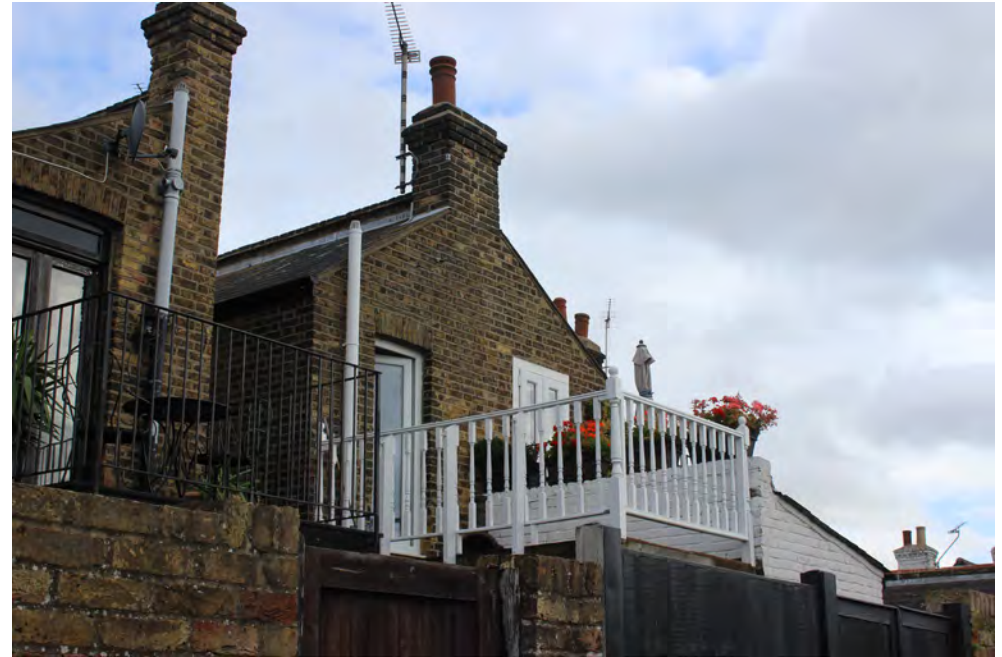
uPVC units on rear elevations of Theobalds Cottages visible from Alley Dock
