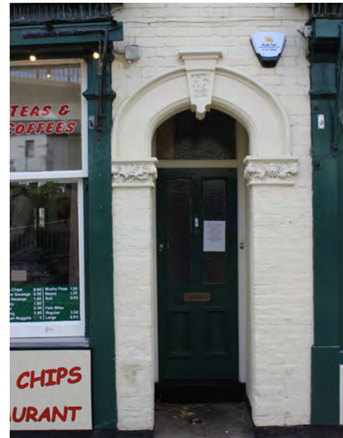
The retained shopfront is negatively impacted by pigeon deterrent spikes, redundant lights and plastic signage
